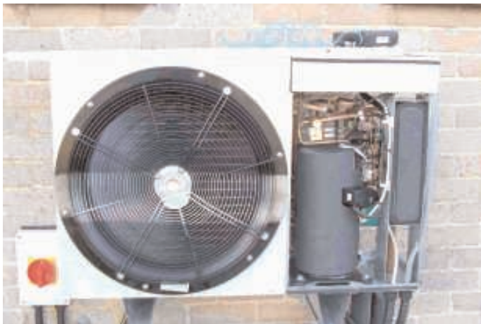
Heating B-Warm Air Source Heat Pump
